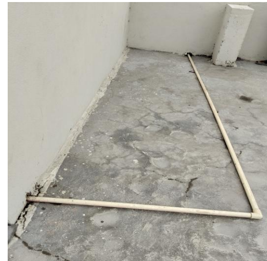
After filtration, the wastewater flows out through this pipe
