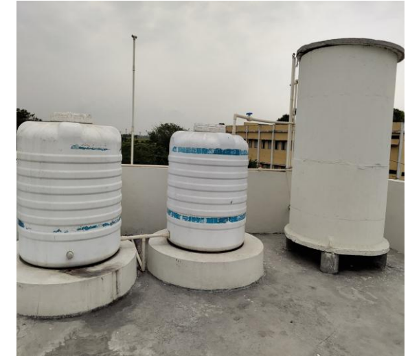
Tanks for storage of water for regular use
