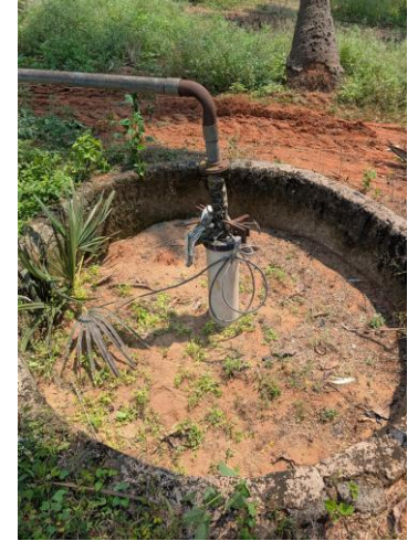
Injection Well for Water Recharge
