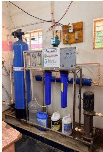
RO Water plant provided to the school
